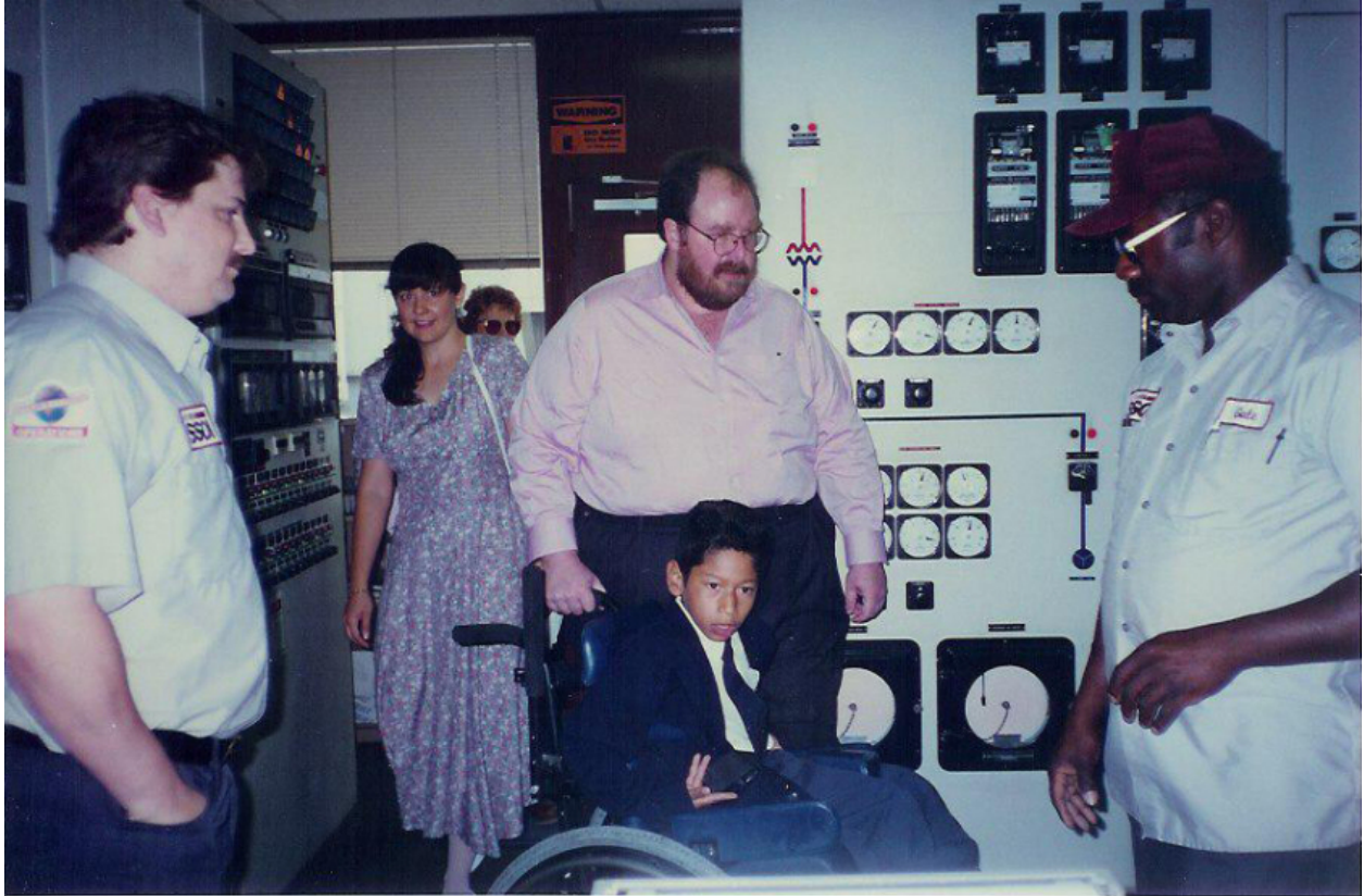
Figure 3 Control room at Growers Cogeneration Plant with friends from Vernon Elementary School and plant operators
