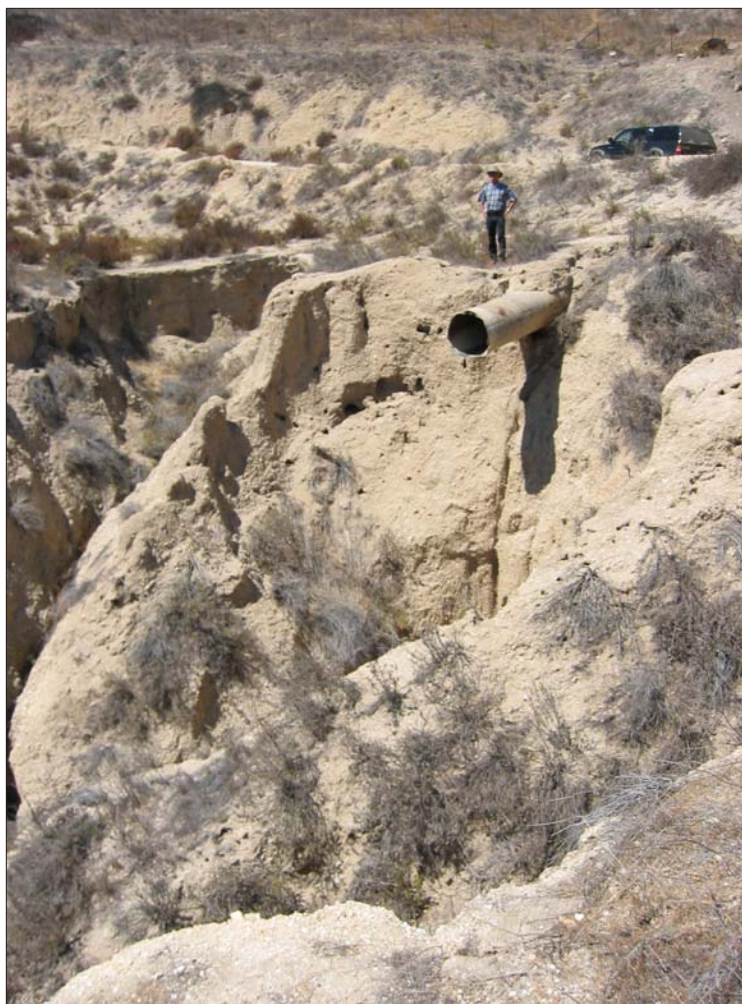
Figure 38. Impacts of culvert on the Tank Road (Source: US-LT RCD, 2007)
