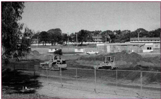
Excavation work has begun for CSUMB's new swimming pool complex. Located near the west side of the stadium, alongside the soccer field parking lot, the facility will feature a 25 meter by 25 yard outdoor pool. A 5,000-6,000 square foot structure will house changing rooms, lockers and mechanical support equipment. It's expected to open during fall 2003.
