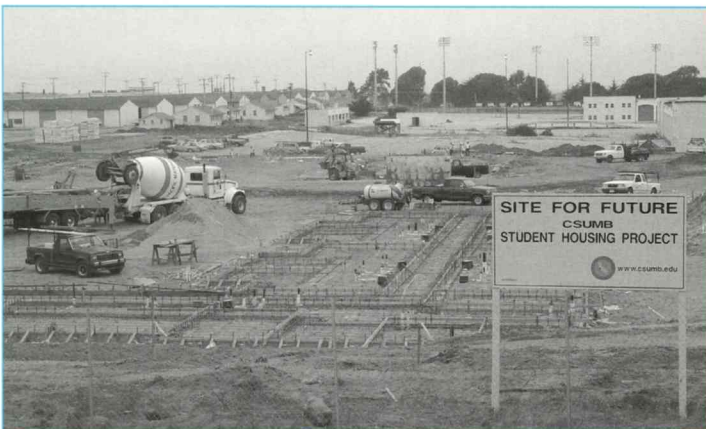
The pouring of concrete foundations for the North Quad student housing project is well underway.
