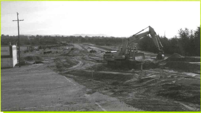
The "old" Second Avenue has been demolished and barricaded at Lightfighter Drive and Imjin Parkway.
