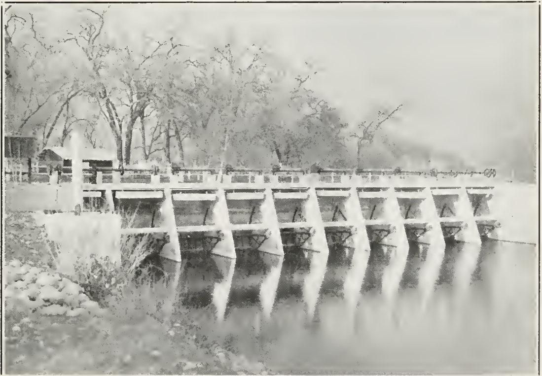
FIG. 2. Headgate of Consolidated Canal on Kings River, Consolidated Irrigation District.
