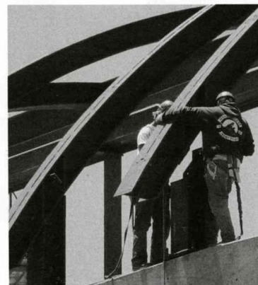
Each 38-foot long steel beam spanning the atrium weighs almost two tons.
