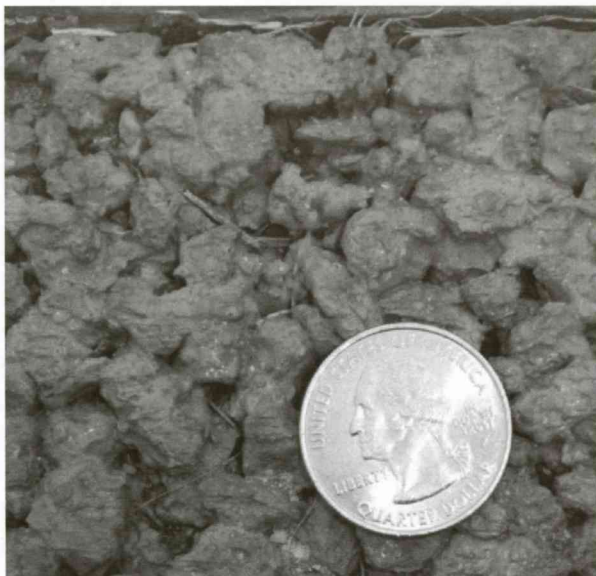
A close look reveals crevices in the pavement that allows water to migrate into the soil below.
