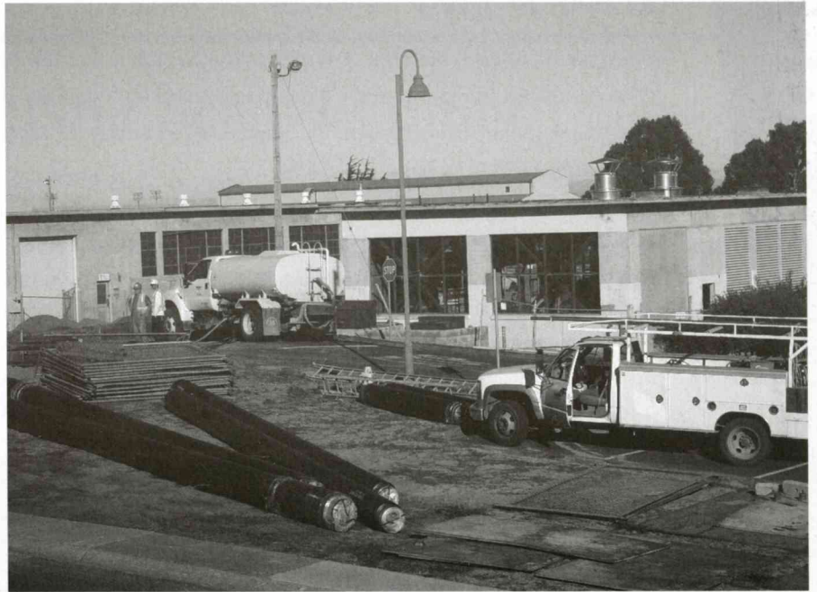
The new central plant (Building 74), located on Inter-Garrison Road adjacent to the Visual & Public Art buildings, will soon provide hot water to heat buildings.
