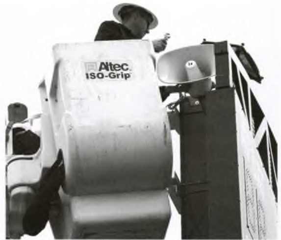
Lloyd Eads, electrician in Facilities Services and Operations, installs an alarm speaker atop baseball field scoreboard. A small solar array is on top.
