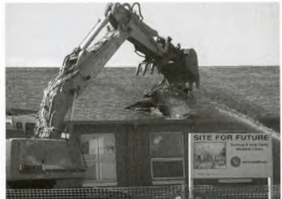
Following demolition of the site in September 2006, a groundbreaking ceremony took place a month later.
