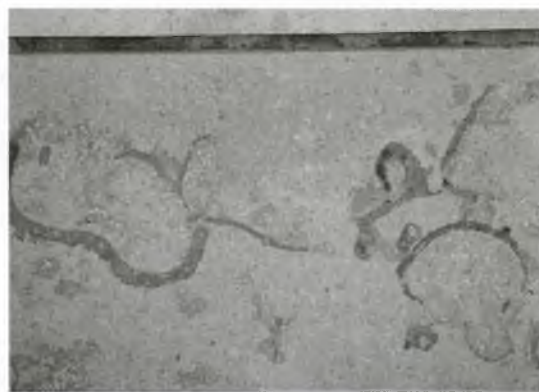
Limestone walls covering the new library's entry facade reveal fossils from millions of years ago.
