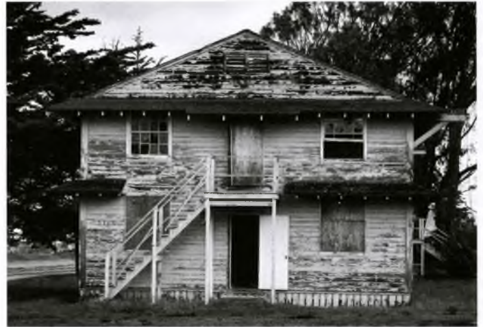
One of five abandoned World War II-era Army barracks near the intersection of Divarty Street and Second Avenue that are being removed.
